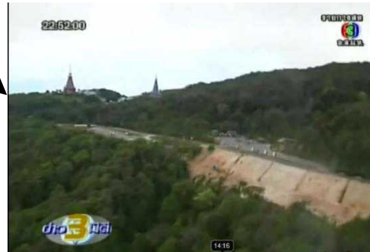
Localised slope failure (highway slope)
