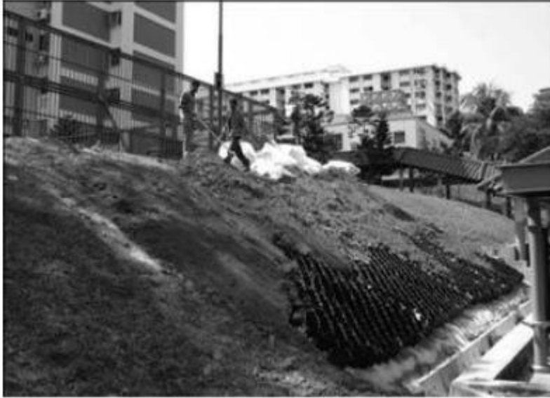
(a) Placement of top soil on top of the fine-grained layer of the capillary barrier system
